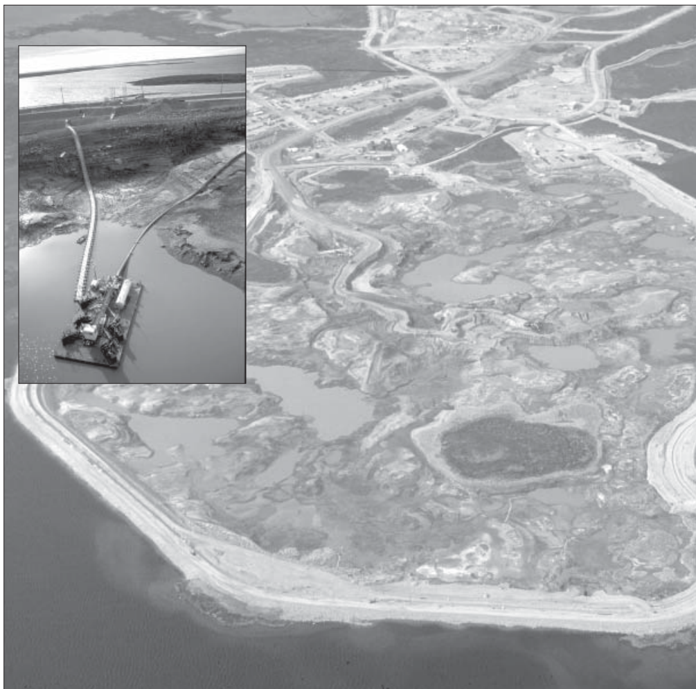
Some 11 million cubic metres of water were pumped from within the A154 dike to Lac de Gras and on-land storage areas. Inset is the south barge.
