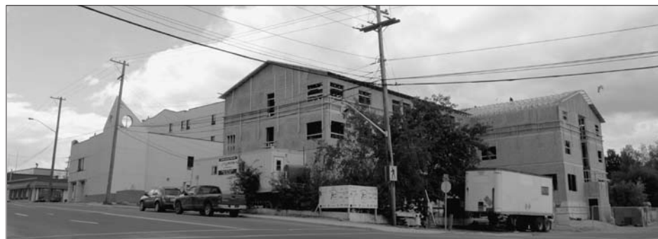
Construction of Bailey House is advancing as planned. The Salvation Army, located next door, will deliver the new facility's programs.
