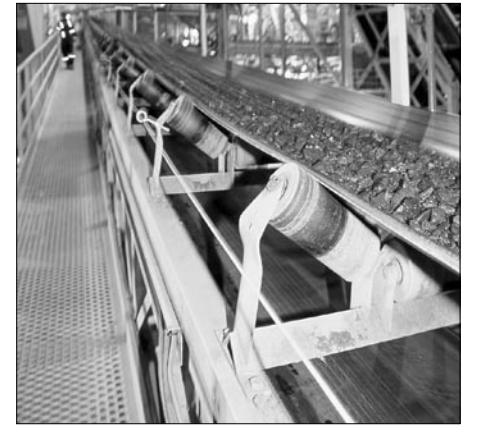
Diamond-bearing kimberlite ore from the plant's re crush circuit is conveyed to the secondary scrubbing circuit.
