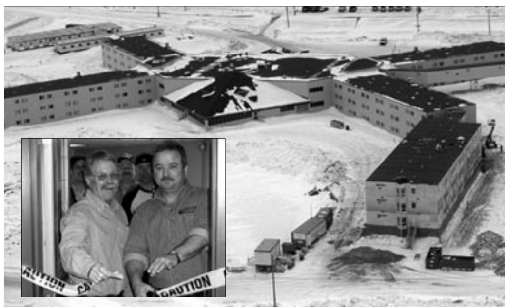
Ekati Travco, a Yellowknives Dene joint venture, completed the 69-room expansion to Diavik's accommodation complex. Inset are Bob Davies of Ek'ati Services, left, and DDMI's Duke Vetor cutting the ribbon to open the addition.
